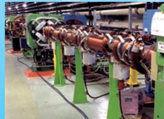
Solenoid magnets for positron ring: Solenoid magnets are installed over the entire positron ring to suppress the harmful build-up of electron clouds. KEKB showed a dramatic increase in luminosity after their installation.
